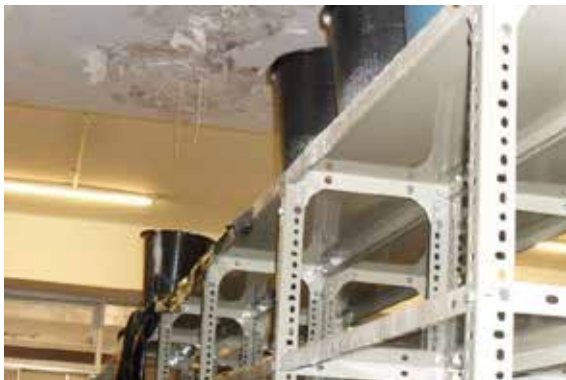
Figure 7: Roof leaking fourth floor stack room 2012
