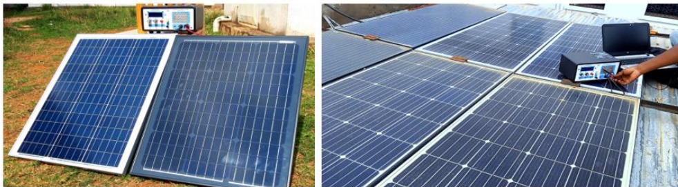
Figure 7: PV module test set-ups: 50 W polycrystalline modules (left) and 150 W polycrystalline modules (right)
