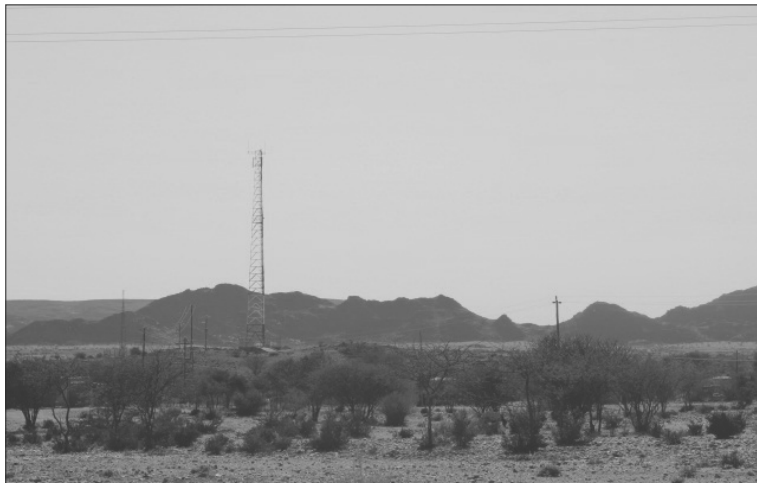
Above: An MTN cellular reception tower built in 2010 in Riemvasmaak Photographic source: Lauren Marx
