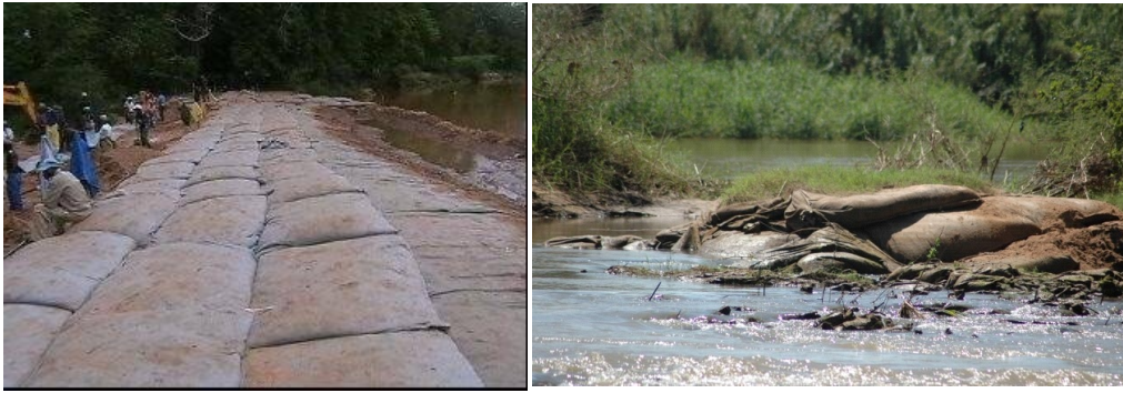
Figure 2: Sand-filled hessian bags stacked to plug the breach in the river bank (A), and displaced sandbags at the breach point following the first spring rains (B). 40
