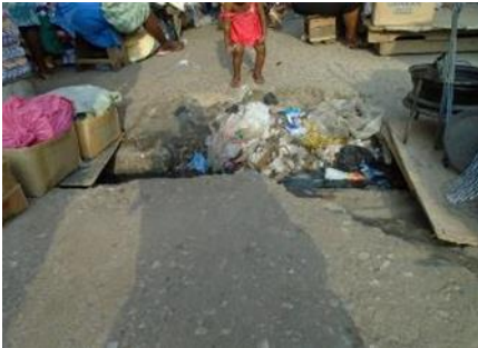
Figure 7: Gutter in the middle of the road in a market
