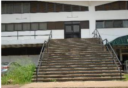
Figure 9: Inaccessible entrance to a classroom
