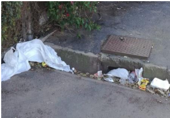
Figure 2: Litter in the drainage system outside the station (Source: Researchers)
